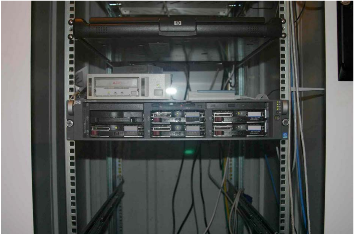
Rack - Server Bünzmatt II
